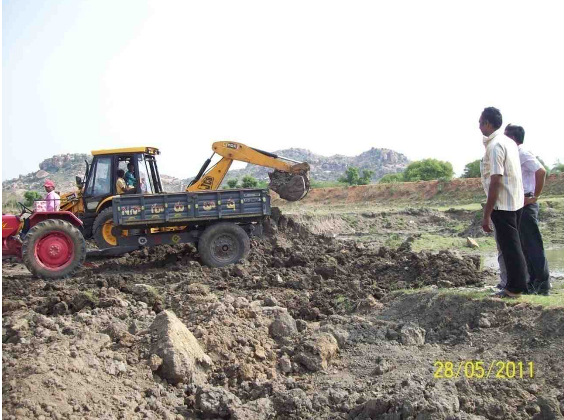
Tank silt applied to enhance soil fertility and increase water harvesting capacity of tanks in Kadapa, Andhra Pradesh
